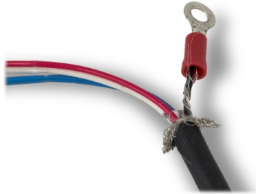
Figure 2-81: Ring Terminal Crimped onto Black and Drain Wires
