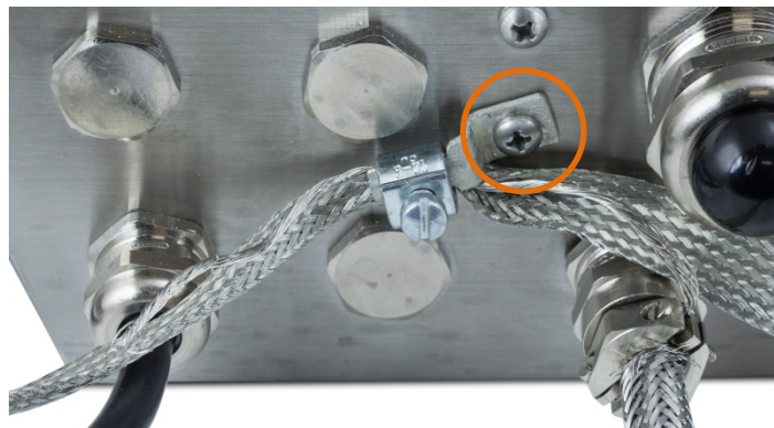
Figure 2-56: Grounding Clamp Mounted to Enclosure
